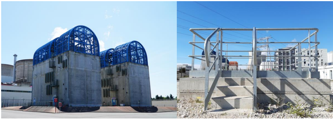
3-MWe station blackout diesel generators [DUS]
